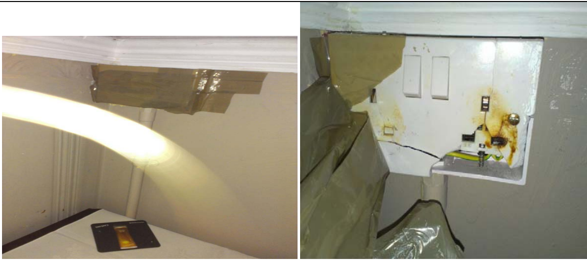
1) Smashed socket cover with signs of burnt electrics
