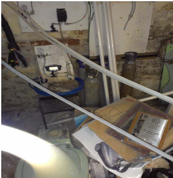
6) Further cluttered and untidy cellar areas with high pressure CO2 cylinders left unchained.
