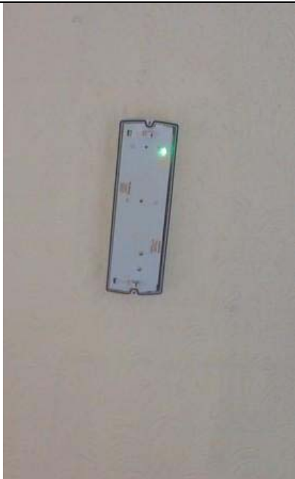
An emergency light with no light bulb in it
